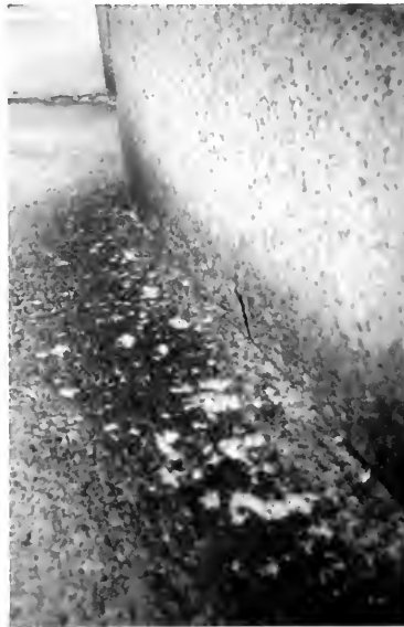
Figure 32: Damaged granite base of pedestal (Photograph by author, March 2002)
